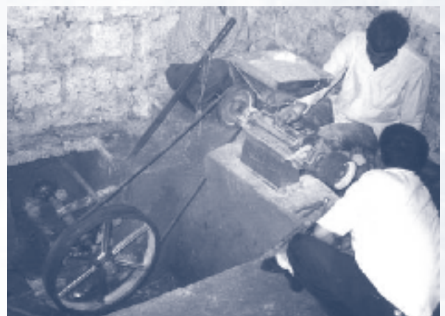
Inside of 5kW micro-hydro powerhouse used for rice milling, Uttarachal, India (©IT Power)
