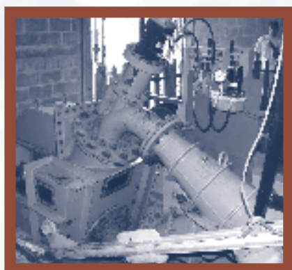
230kW mini-hydro scheme for village electrification in Nicaragua (©IT Power)
