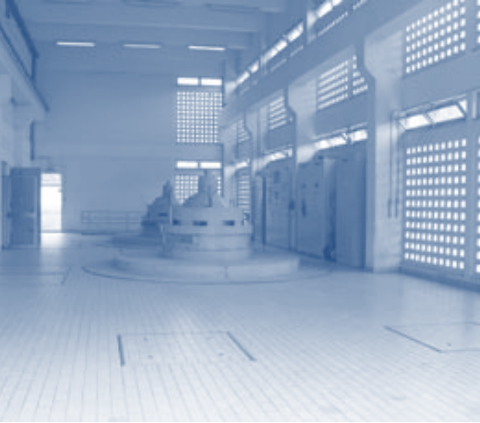
Generators shed, Mukngwa, Rwanda. (© MHyLab)
