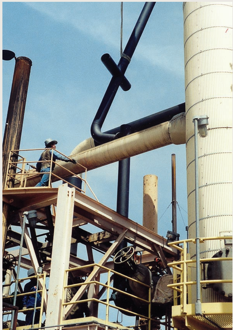
Installation of a PPS-coated steam vent at Cove Fort in Utah.
