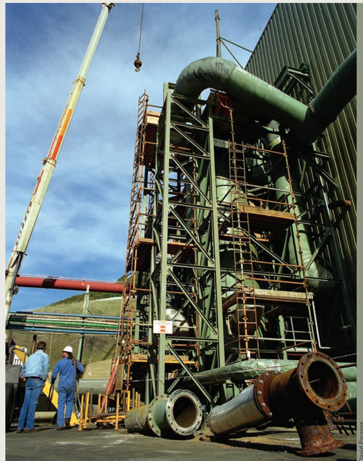
Condensers being retrofitted with direct contact condensers at The Geysers Geothermal Power Plant in California.
