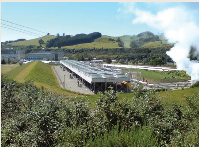
The Wairakei Geothermal Power Plant in New Zealand.
